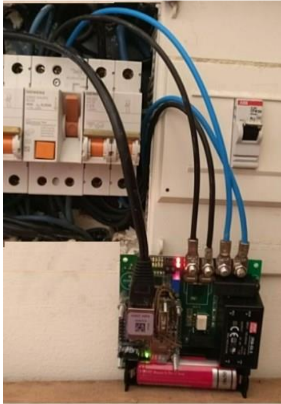
Figure 2 Installation of oZm in the electric panel of a building.
