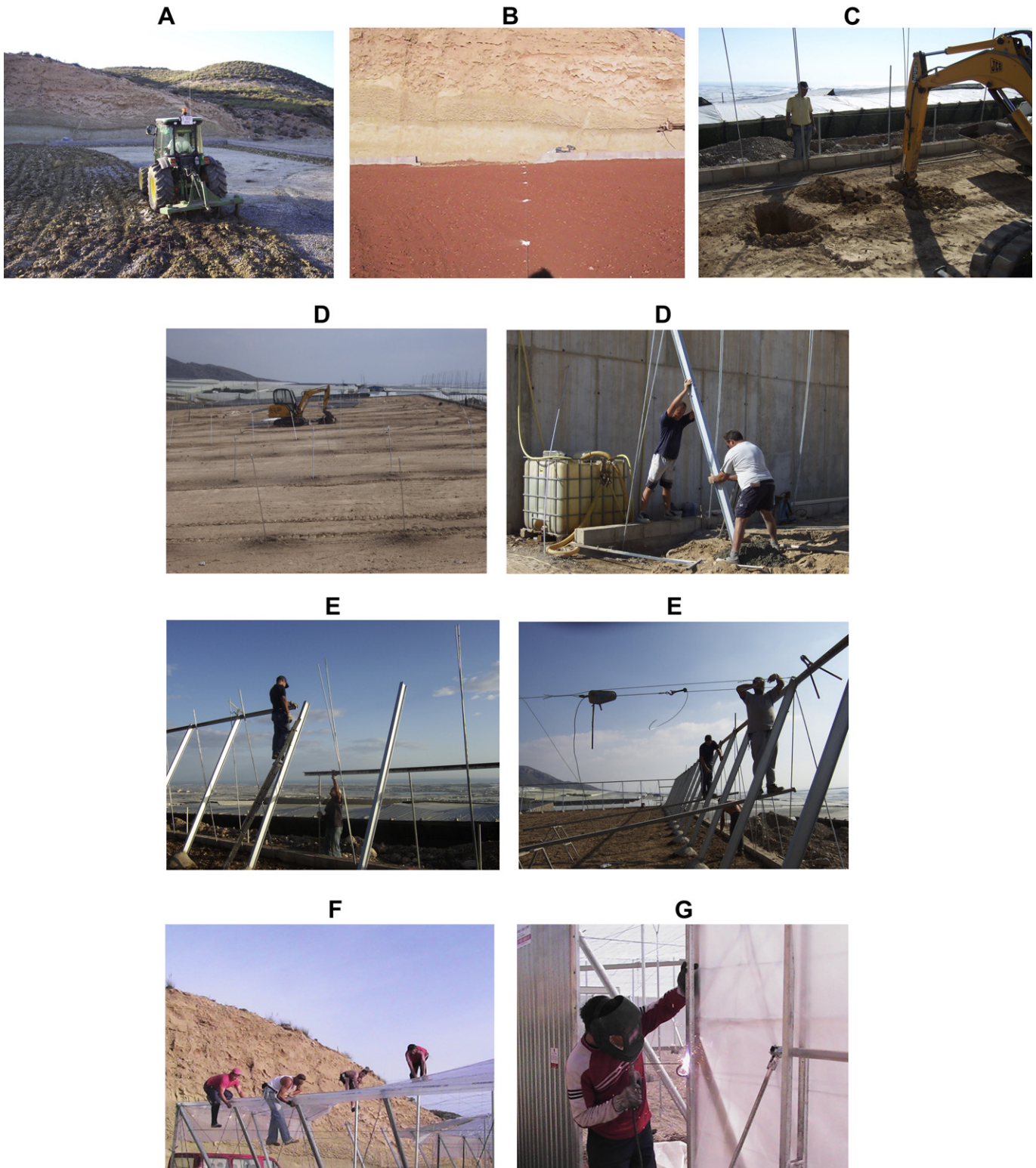
Fig. 1. Stages of the greenhouse-construction process: (A) Weed clearing, land levelling, and soil preparation, (B) replanting, (C) digging and perforation of holes for the foundations and anchors, (D) foundations and anchors, (E) building of the structure, (F) placement of the plastic and (G) installation of windows and doors.
