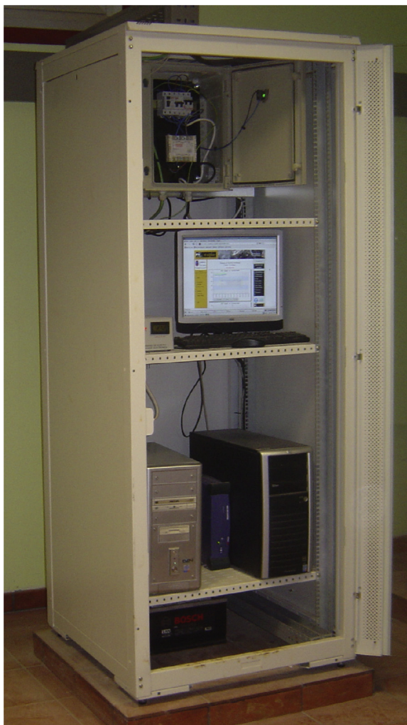
Fig. 6. Closet of the central control station.
