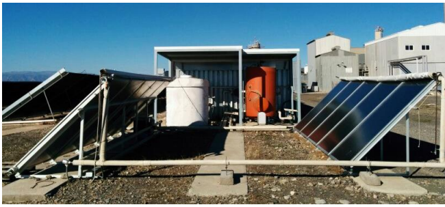
Figure 2. Solar facility at PSA.
