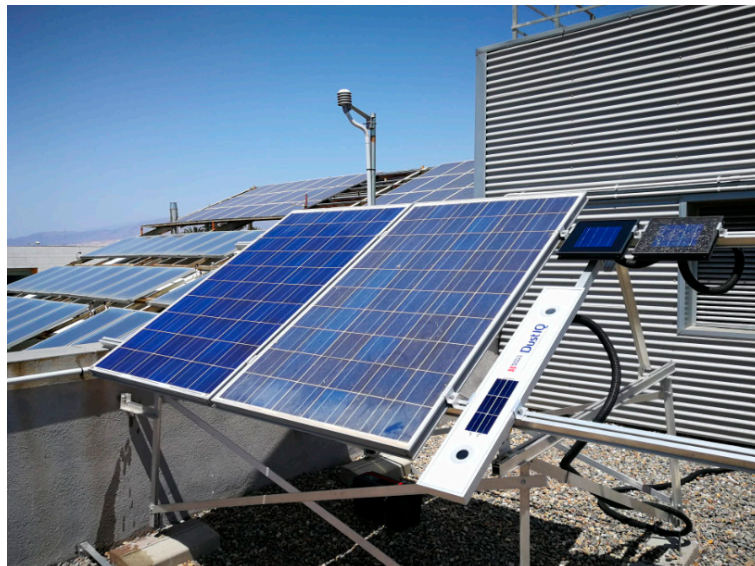
Figure 1. Monitored experimental installation.
