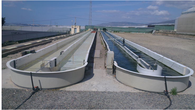
Fig. 1. Real view of the raceway photobioreactor.
