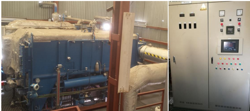
188 Figure 2. DEAHF LiBr-H 2 O facility at the PSA on the left and the programmable logic 189 controller on the right 190
