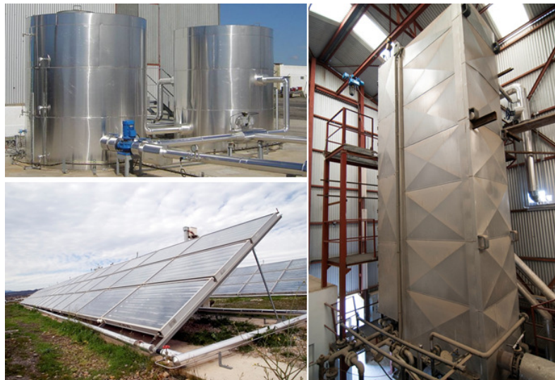
Figure 2. Solar desalination facility at PSA-CIEMAT. From left to right and from top to bottom: cold and hot tanks, MED unit and solar field.
