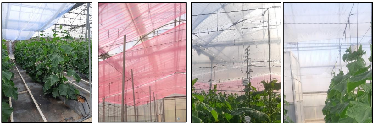
Figures 1a, b, c, and d. Experimental Blue, Experimental Pink, French-Standard, and Almería-standard plastics, respectively, installed in experimental Multi-tunnel greenhouses.
