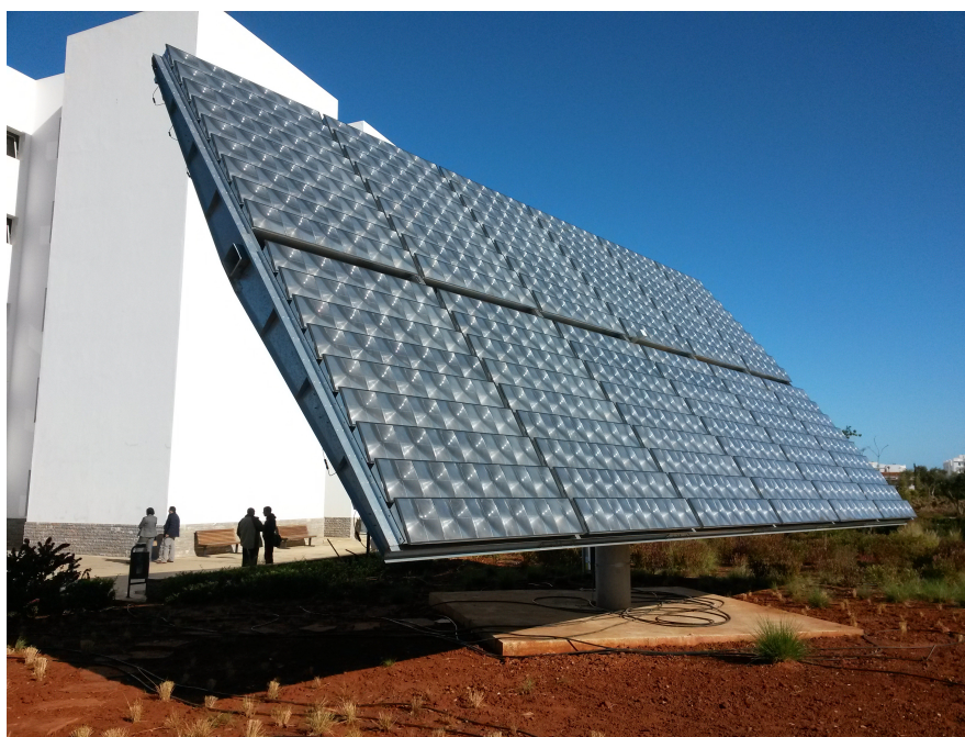
Figure 2. The high concentrator photovoltaic (HCPV) facility used in this work.
