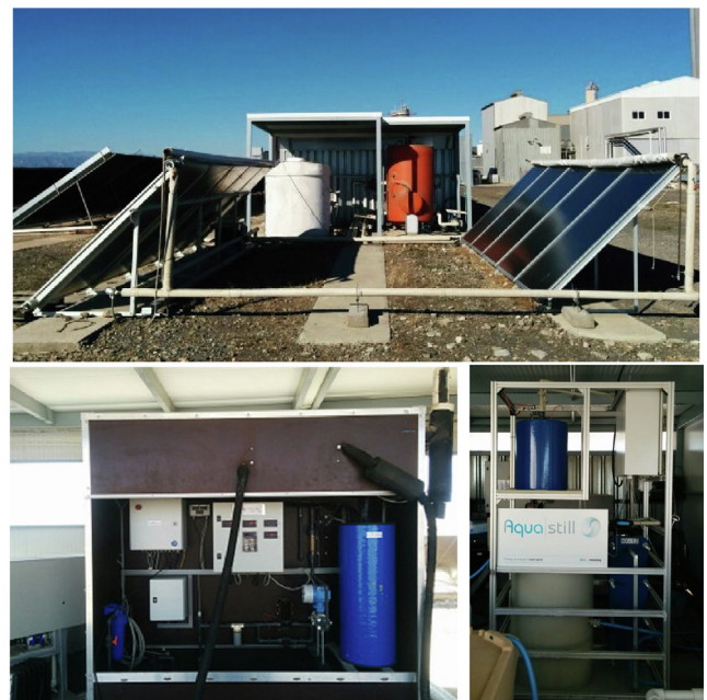
Fig. 2. SMD pilot plant at the PSA. From top to bottom and from left to right: the solar field, the Solar Spring module and the Aquastill module.
