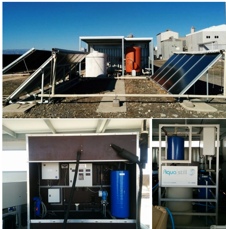
Figure 1.5: SMD pilot plant at PSA. From top to bottom and from left to right: solar field, Solar Spring module and Aquastill module.
