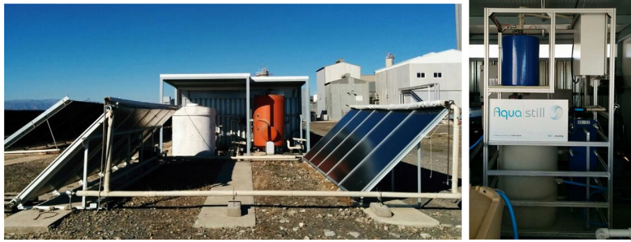
(a) SMD facility. (b) Aquastill pilot module.
