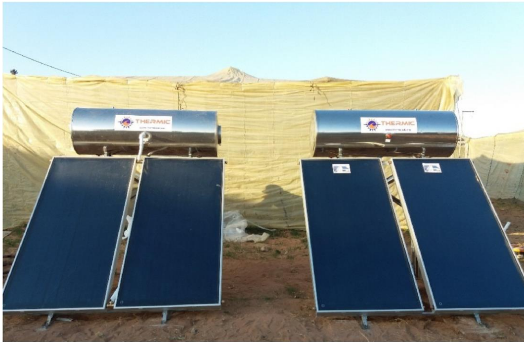
Fig. 2. Thermosiphon thermal solar collectors with water closed-circuit and 300 L of storage volume.
