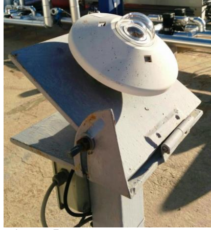
Figure 5. Pyranometer at the PSA
