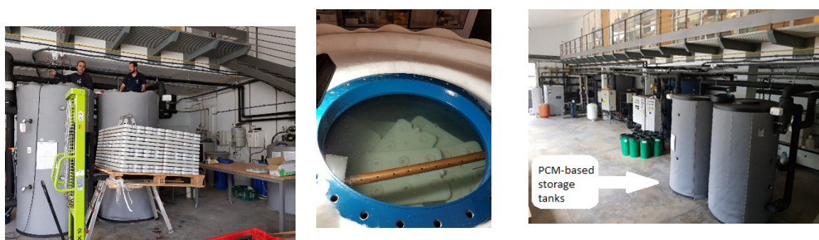
Figure 13. The SCH system with two newly installed PCM-based storage tanks.
