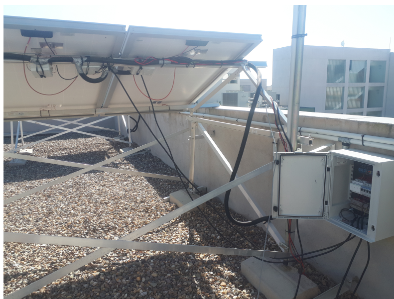
Figure 6. UHU-MUX multiplexer installed at the experimental PV facility of the Universidad de Almería.
