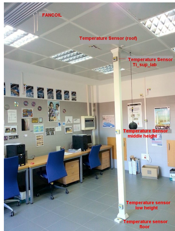
Fig. 2. Laboratory 8: the location of temperature and fancoil sensors.
