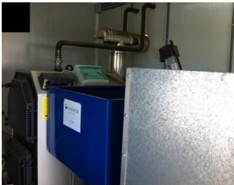
Figura 2.21 Caldera Biomasa Missouri 150 KW [40]
